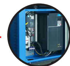
VSD Controller for Main & Fan Motor
